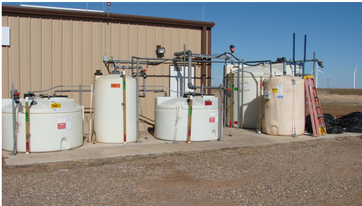
FIGURE 8.5 — Chemical Injection Tanks
