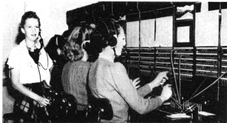
Pictured above are some of the telephone operators at work on the four position switchboard. They are, seated, right to left, Gertrude Carroll, Jimmie Lee Hafen, Rosella McQueen, and Margaret Chance. Standing is Supervisor Jewell Kolb.
