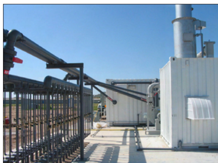
Zone 11 SVE system
