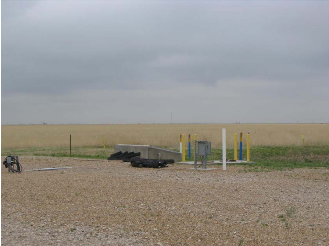
Southeast In-Situ Bioremediation System (SEISB) Equipment Pad (with electrical and injection distribution connections for the Injection Trailer)
