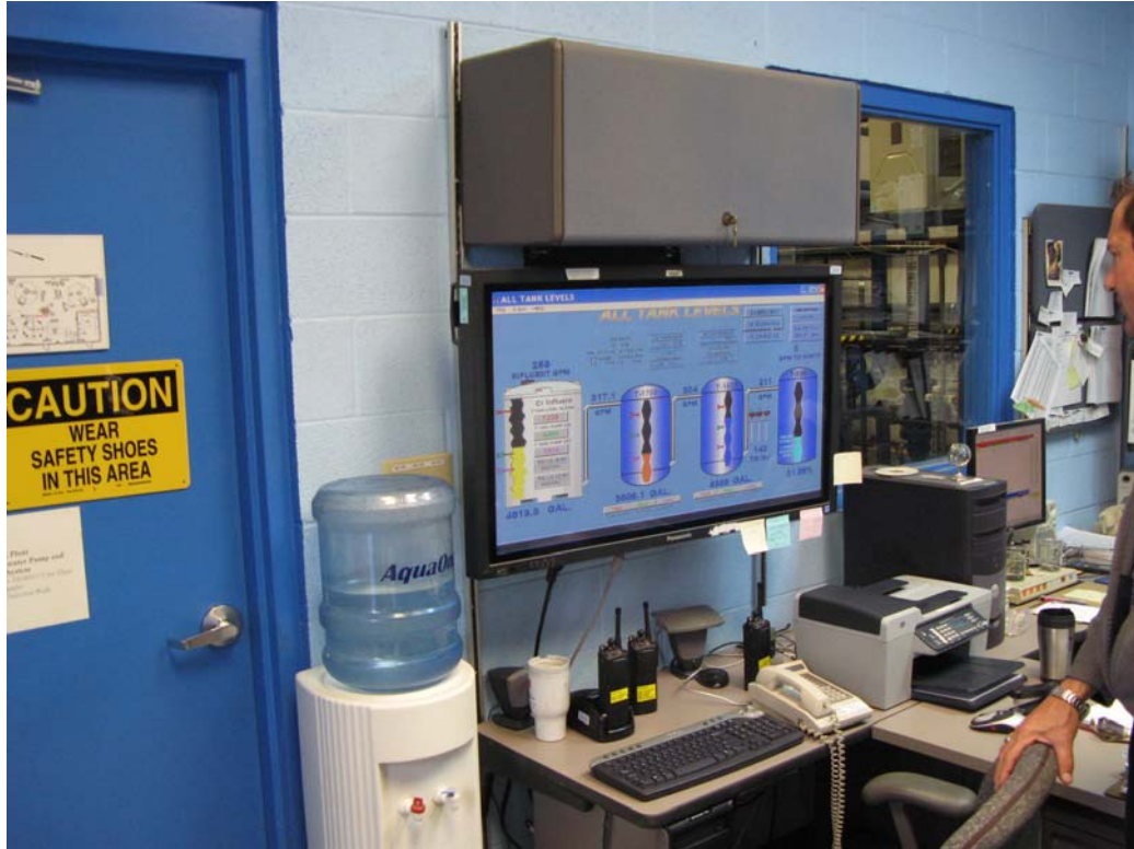
Southeast Pump & Treat System (SEPTS) Control Room
