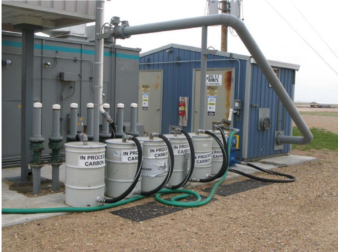
Burning Ground Soil Vapor Extraction System (with GAC Canisters in the foreground)
