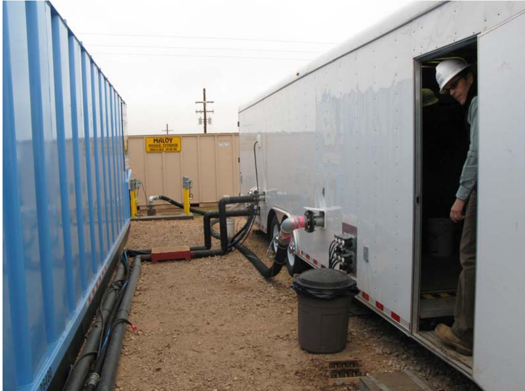
ISB Injection Trailer
