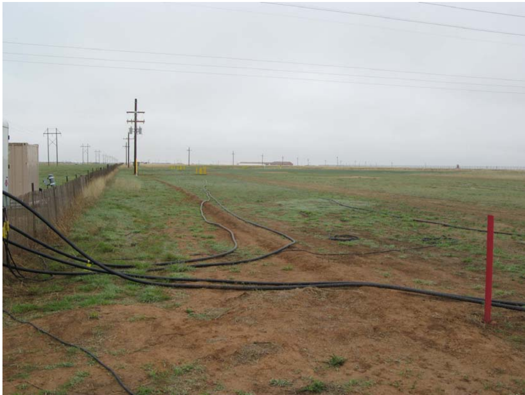
Black Hoses Carrying Amendment to the Injection Wells at the Zone 11 ISB
