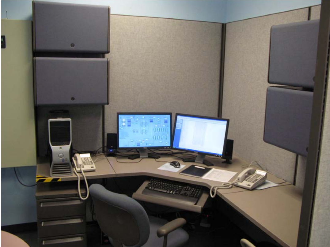
Playa 1 Pump & Treat System (P1PTS) Control Room
