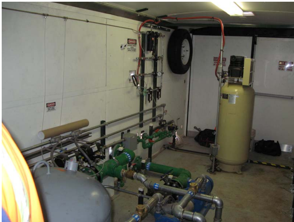
Air Compressor and Inlet Piping for Amendment and Makeup Water Feeds
