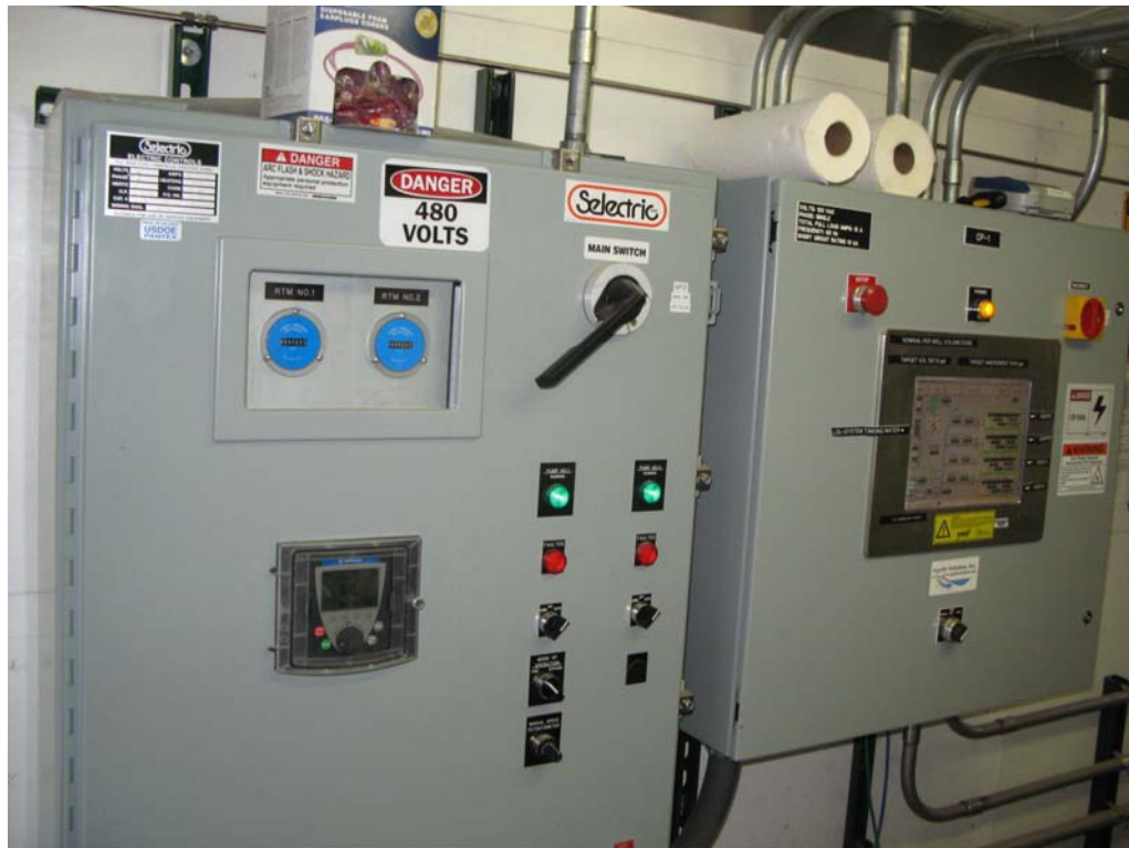
ISB Injection Trailer Control Panels
