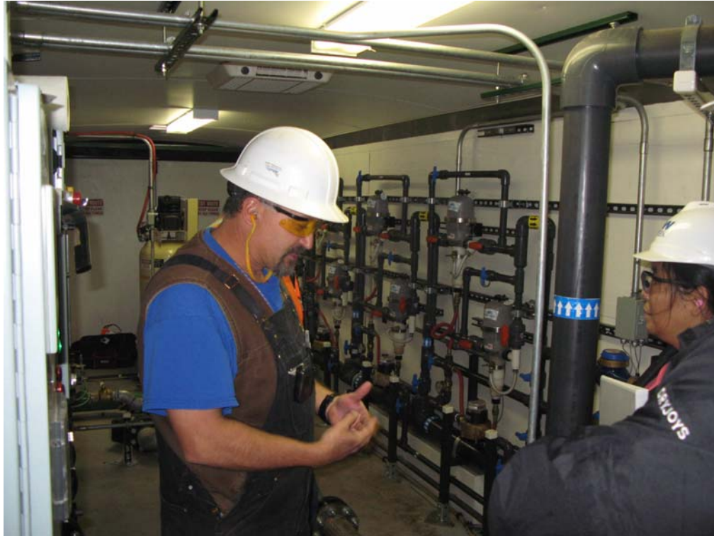
Injection Pumps, Meters, Piping (inside ISB Injection Trailer)
