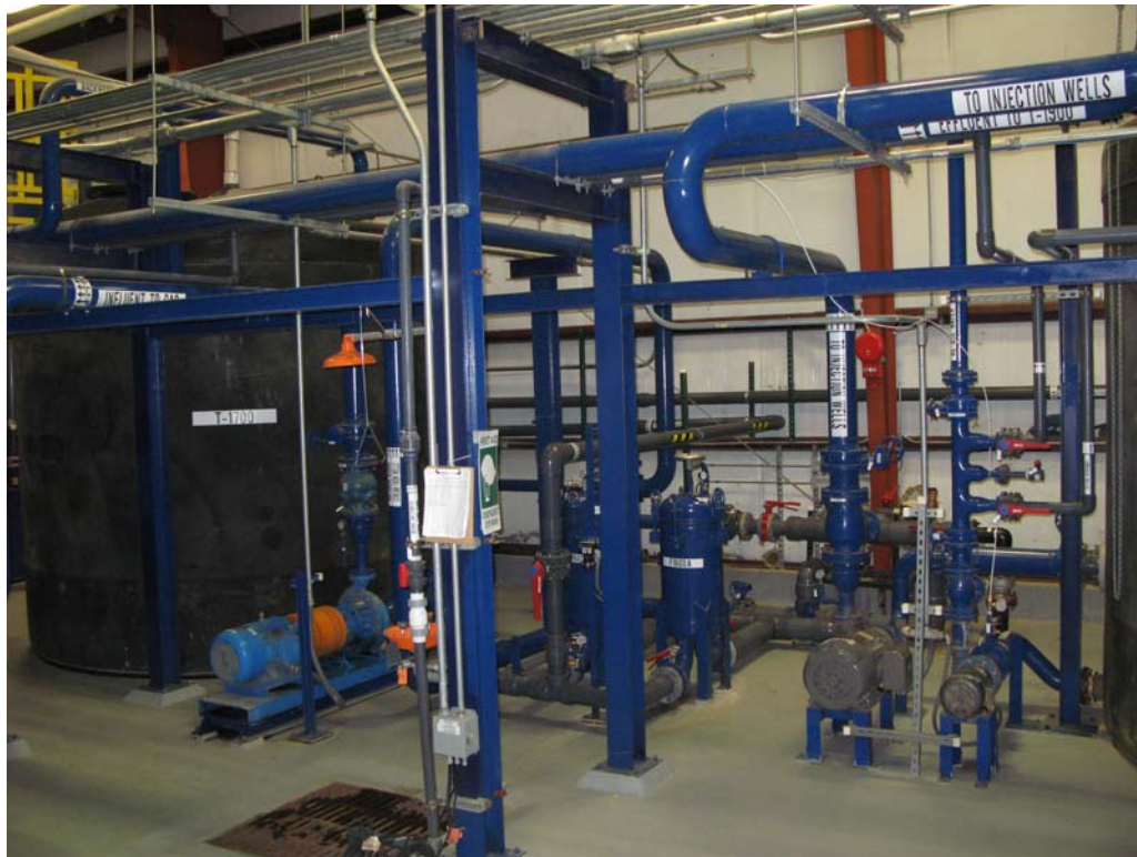
SEPTS Treatment Bay – Pumps & Pre-filters
