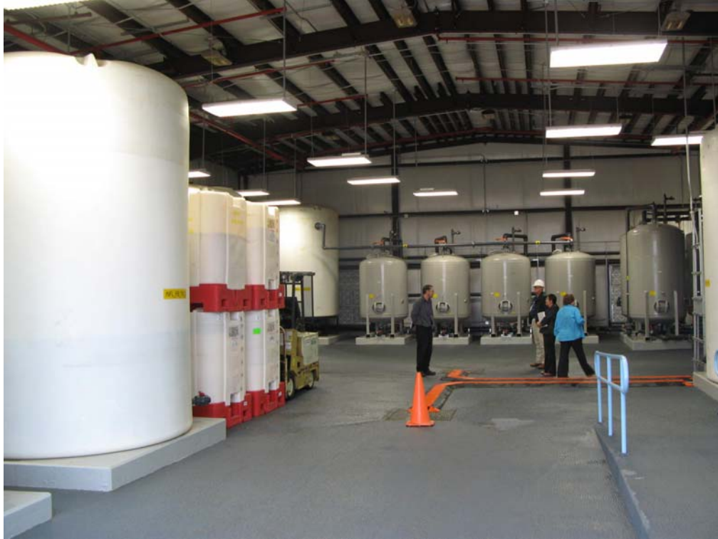
P1PTS Treatment Units (Influent Tanks, IX Resin Totes, Equalization Tank, GAC Vessels)
