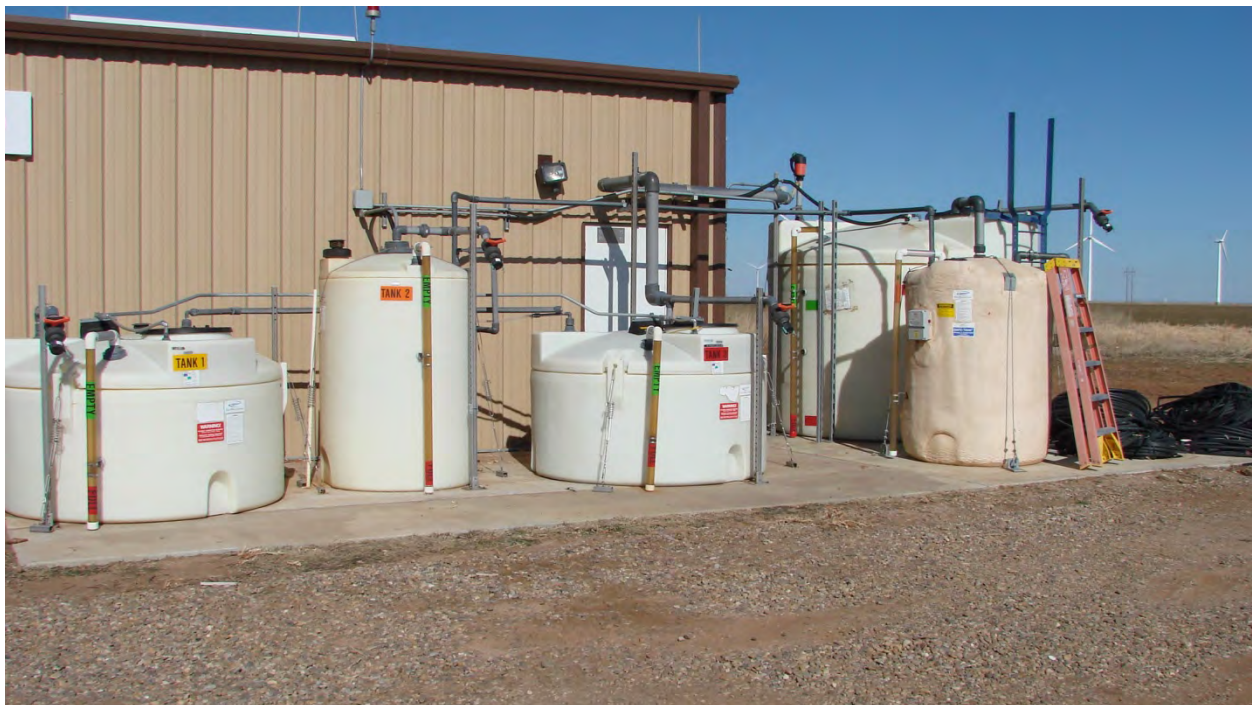
FIGURE 8.5 — Chemical Injection Tanks
