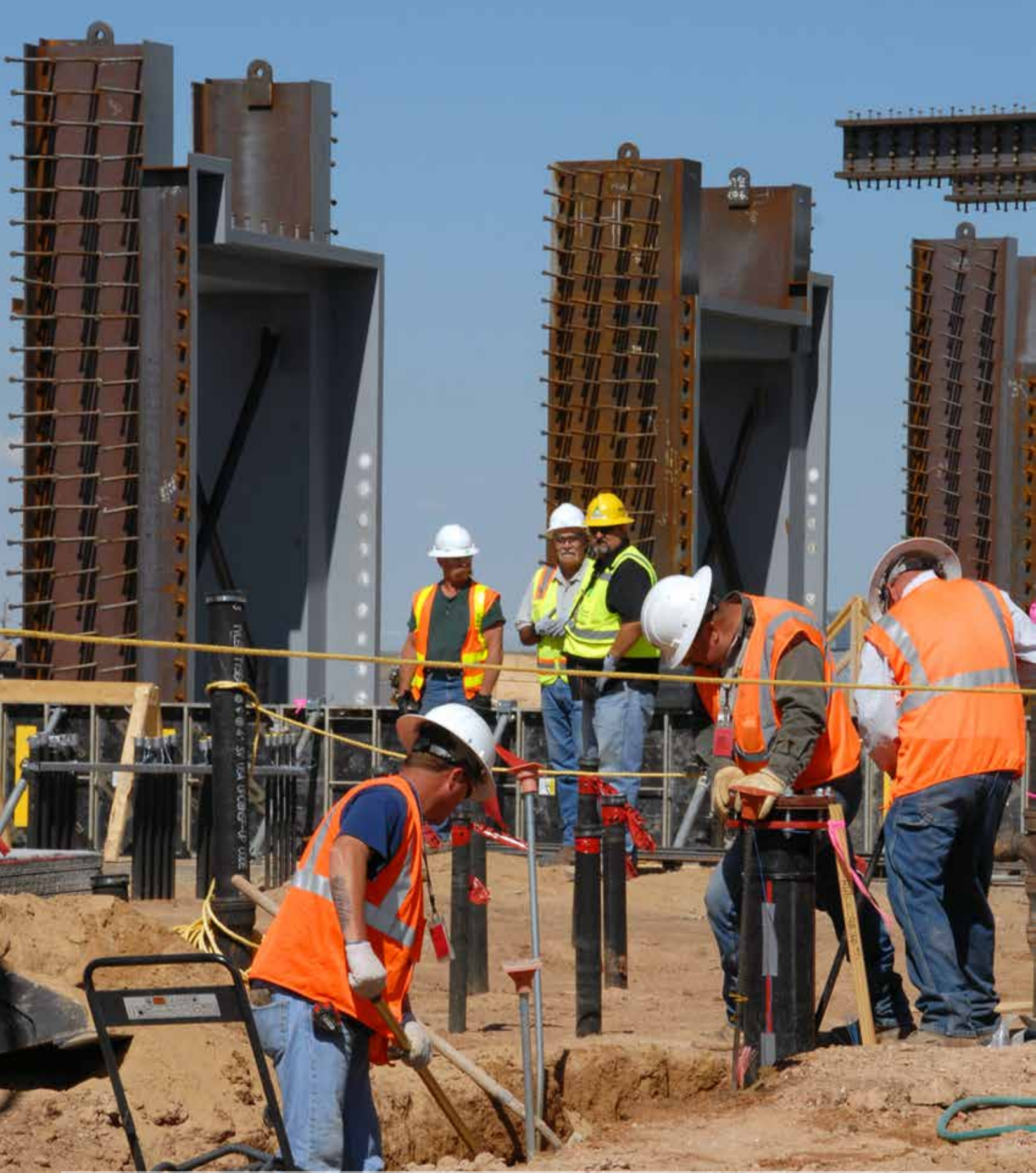
Construction crews prepare to pour concrete at the new High Explosives Pressing Facility project. The project is designed using the 3D Building Information Model approach, an innovation that allows for course corrections and reflects real-time changes in the field. When completed, the HEPF will not only consolidate and improve operations, but increase levels of protection for workers.
