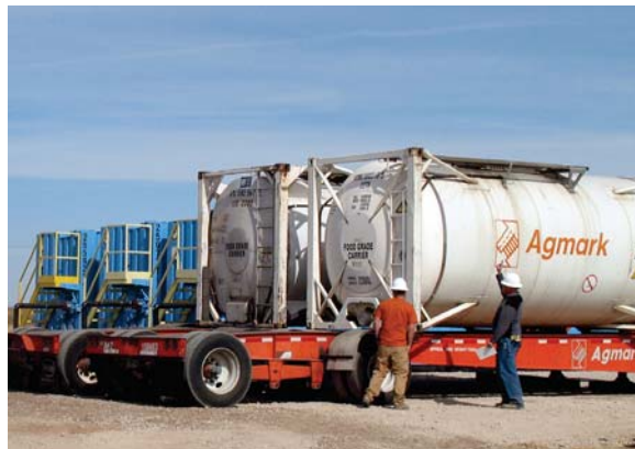
Tankers of food grade amendment to be injected into perched groundwater to create an enhanced anaerobic bioremediation zone.
