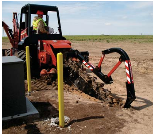
Trenching for a conveyance line to carry water from a new extraction well to the treatment building.
