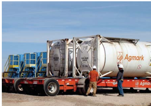
Tankers of food grade amendment to be injected into perched groundwater to create an enhanced anaerobic bioremediation zone.
