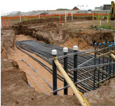
Installation of piping and manifold for a soil vapor extraction system at Pantex.
