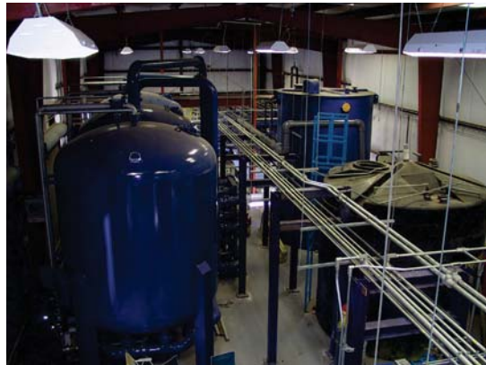
Groundwater pump and treat system at Pantex.
