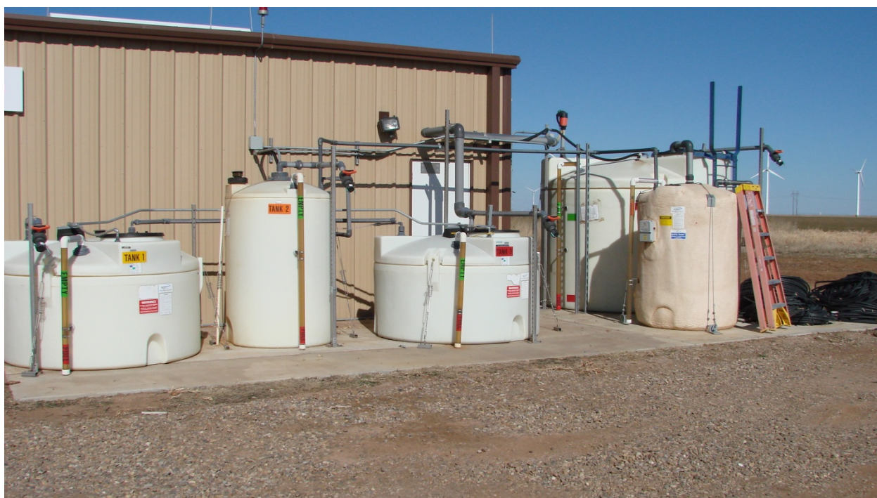
Figure 8.5 – Chemical Injection Tanks
