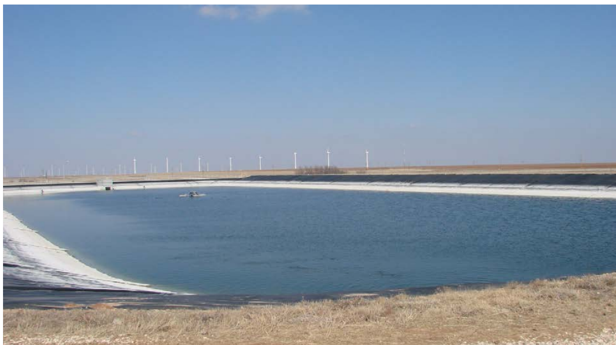
Figure 8.3 – East Wastewater Storage Lagoon
