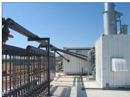
Zone 11 SVE system
